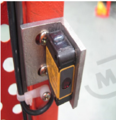
Receiver - No lights on. Indicates no power supply.
