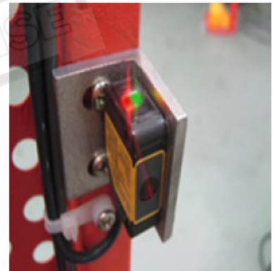
Receiver - Red & Green lights on. Indicates power is on & aligned.
